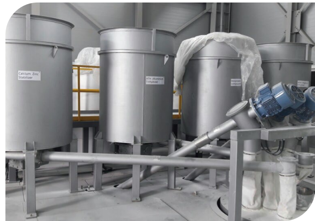
FM Facilities - Material Tank(재료저장탱크)
